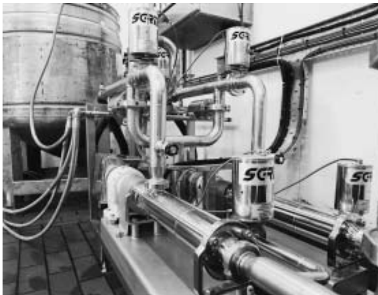
Fig. 3.54 Illustration showing the use of screw type pump to meter fruit from a tank into the yoghurt line
