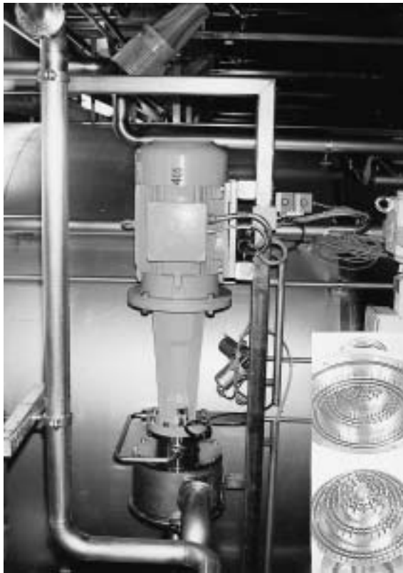
Fig. 3.49 General view of Ytron®-Z “Yoghurt – Stretching” unit on a yoghurt processing plant
