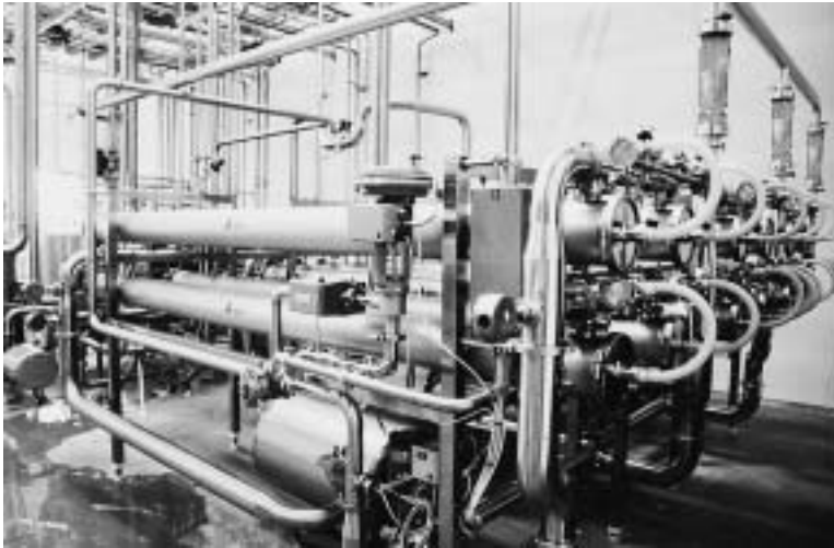
Fig. 3.28 View of an ultrafiltration plant which can be employed for yoghurt production Reproduced by courtesy of APV Nordic, Denmark.
